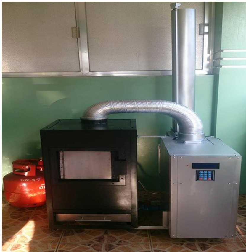
Figure 2. Waste Incinerator with Electrostatic High Voltage Air Filter System
